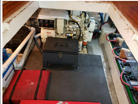
Engine room from saloon deck looking forward to genset
