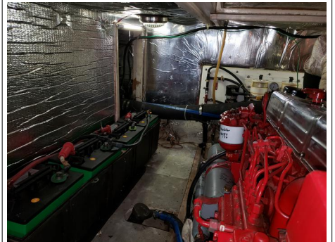
Engine room looking aft starboard side
